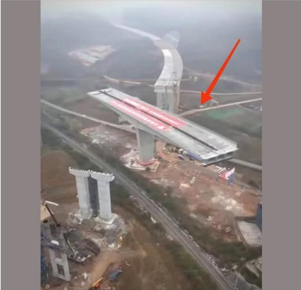
A 169-meter-long, 24,000-ton bridge in Yunnan was rotated and installed over a railway without disrupting train operations. Precision, innovation, and brilliance at its finest
